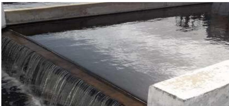
Figure n 14: Bassin de chloration
