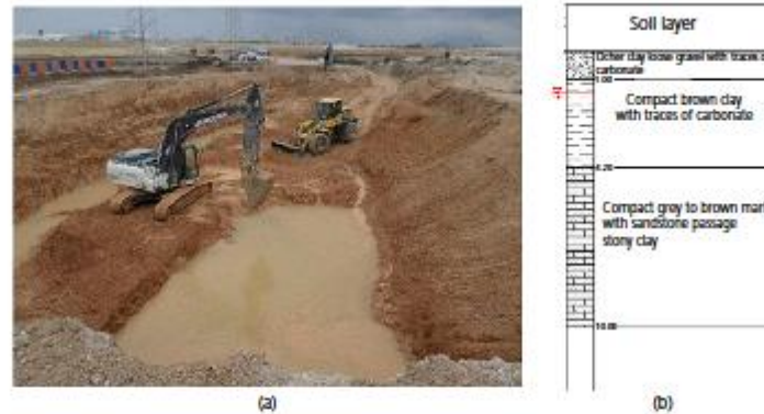
Figure 2. (a) Flooded areas (image provided by Yapi Merkezi Company); (b) the profile of soils at the site of tramway (provided by Algiers Metro Company)
