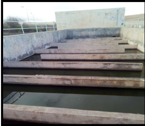
Station de chloration
