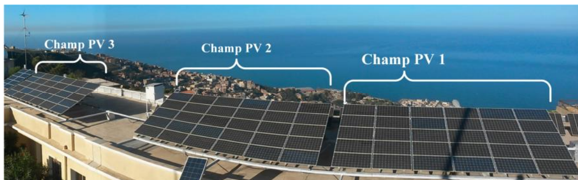
Figure 5.9 : Champ photovoltaïque du CDER
